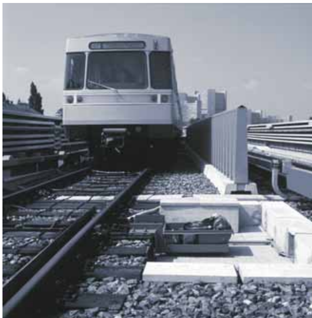
Picture 4: Points Machine along the tracks.
